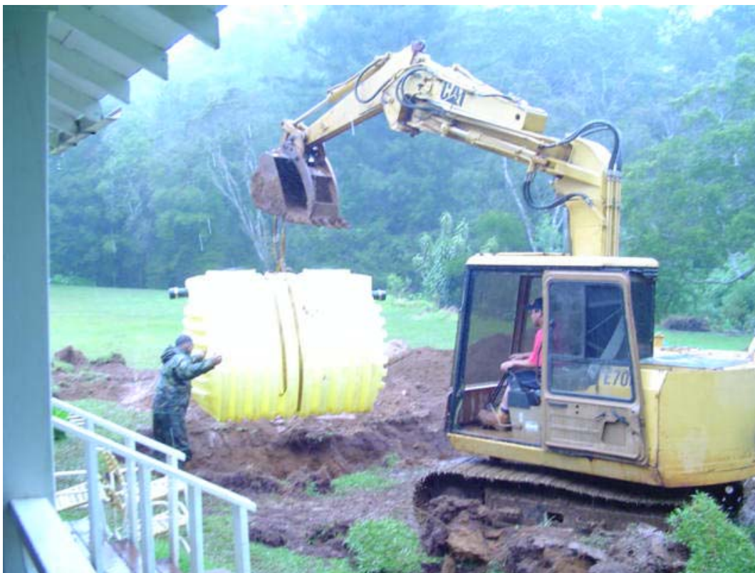
Eddie Molina (left) and Brandon Anakalea (right) – Lowering a 1250 gallon septic tank into the ground at the YWCA Camp Sloggett Lodge, March 5, 2005 – photo by Sharon Ortiz, YWCA of Kauai
